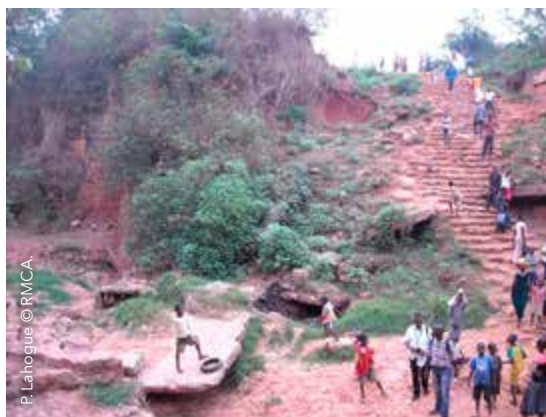
Large sunken area in Mbuji mayi where karst lies beneath a sandstone layer. The path originally lay flat at the top level of the stairs, which were built after the ground collapsed.
